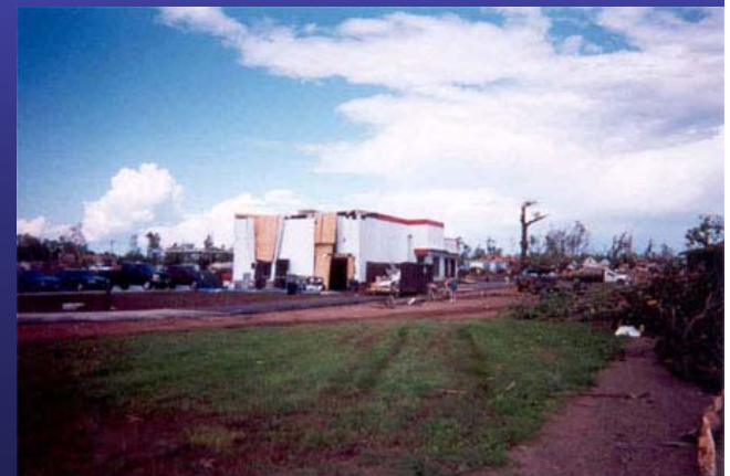
Siren, WI, June 20, 2001 -- An F-3 tornado on June 18 severely damaged the Dairy Queen that had just opened in April. Before the tornado, Burnett County had been under a major disaster declaration for flooding.
